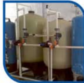
Demineralisation (DM) Plant
