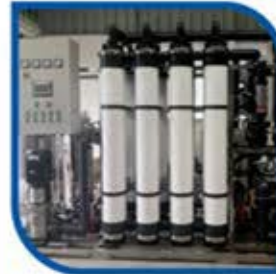
Ultra filtration (UF) System
