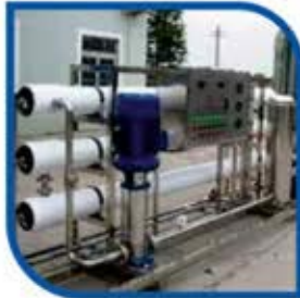
Reverse Osmosis (RO) Plant
