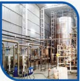
Sewage Treatment Plant (STP)
