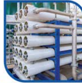
Ultra filtration (UF) System
