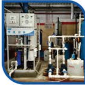
Reverse Osmosis (RO) Plant
