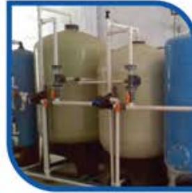
Demineralisation (DM) Plant
